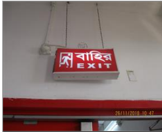
Photo of fire safety equipment Electrical exit sign.JPG
