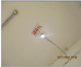
Photo of fire safety equipment Emergency light.JPG
