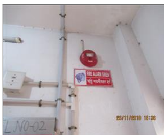
Photo of fire safety equipment Fire alarm.JPG
