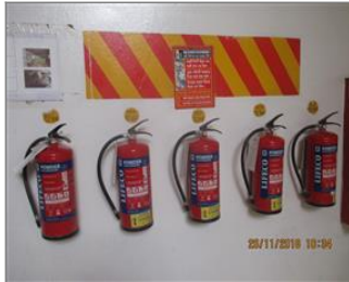
Photo of fire safety equipment Fire extinguishers.JPG
